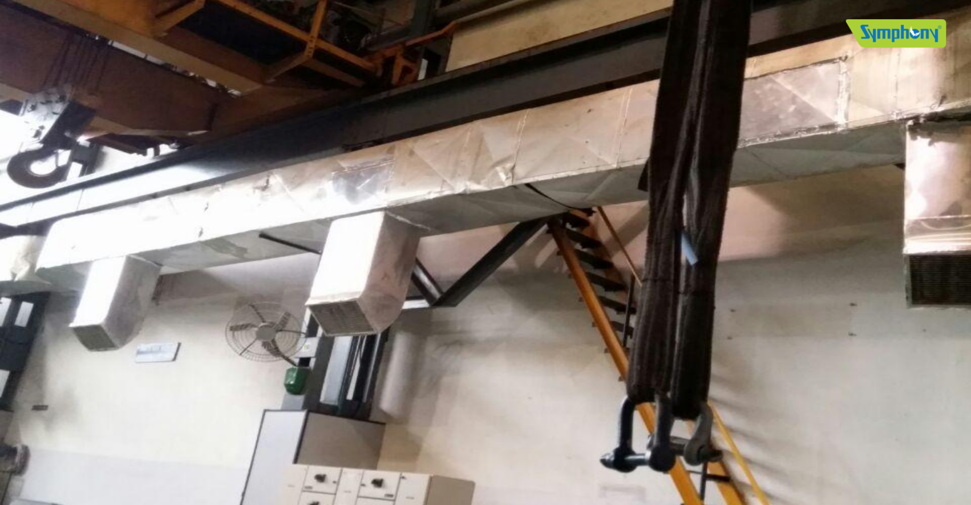
Ducting – All machines are connected to 200 feet duct having 6 to 7 outlets.
