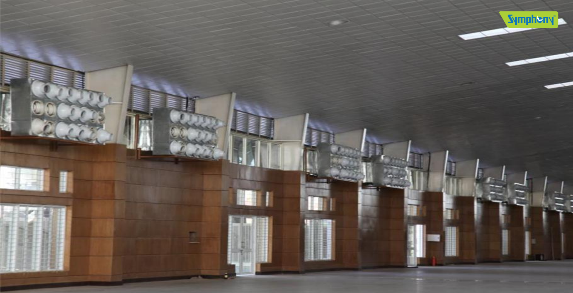
Ducting – All machines are connected to 12 feet duct having 21 Spot Diffusers.
