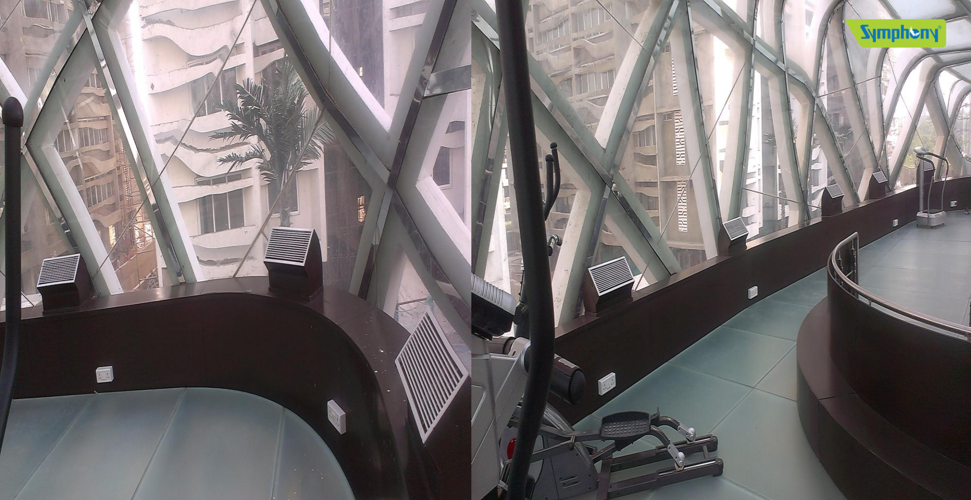
Ducting – All machines are connected to 40 feet duct having 4 to 5 outlets.
