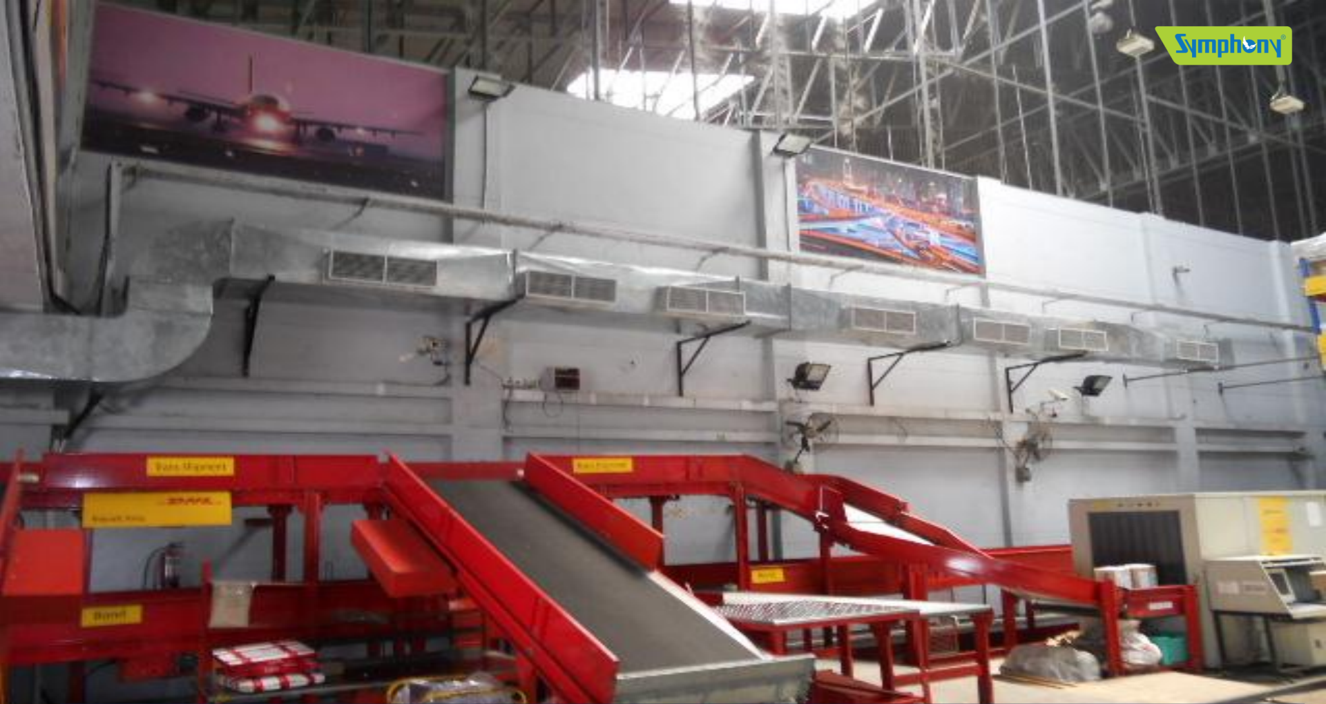
Ducting – Machines are connected to 100 feet duct having 12 to 14 outlets.
