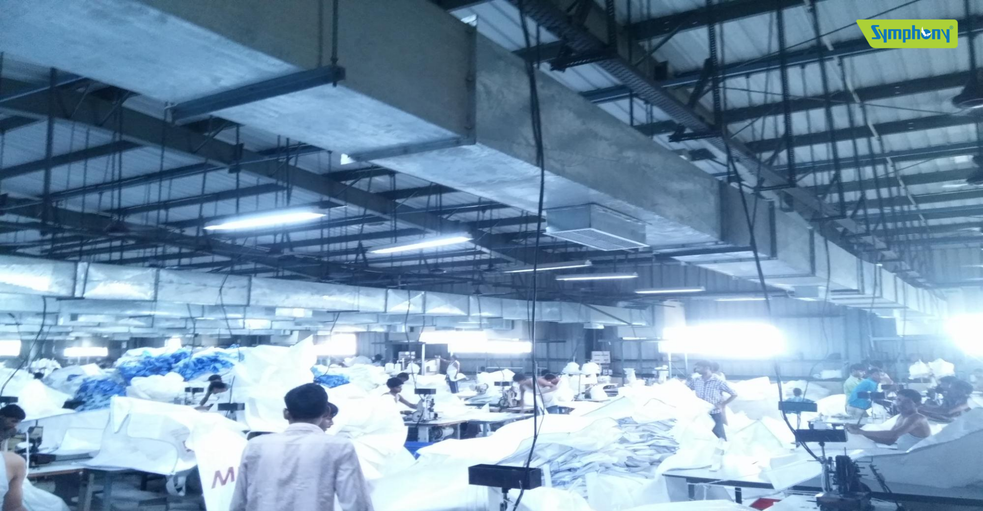
Ducting – All machines are connected to 90 feet duct having 7 outlets.
