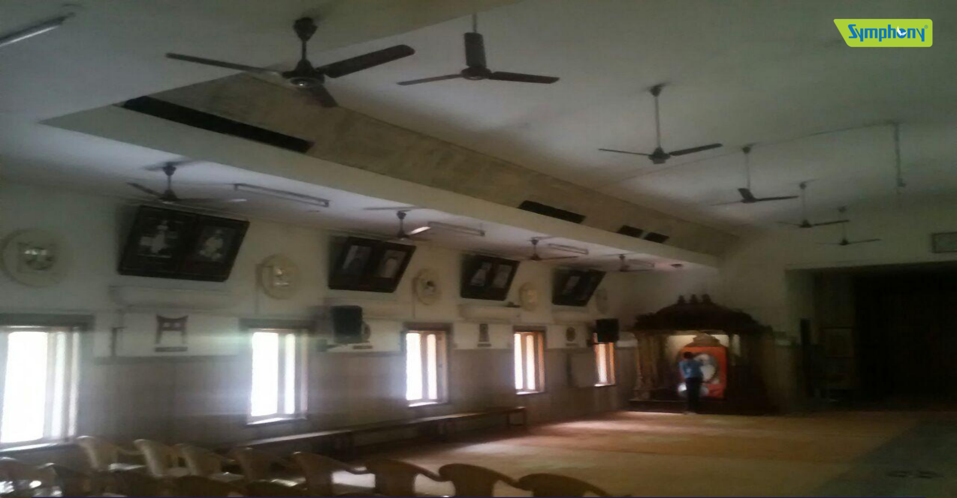
Ducting – All machines are connected to 15 feet duct having 2 outlets.
