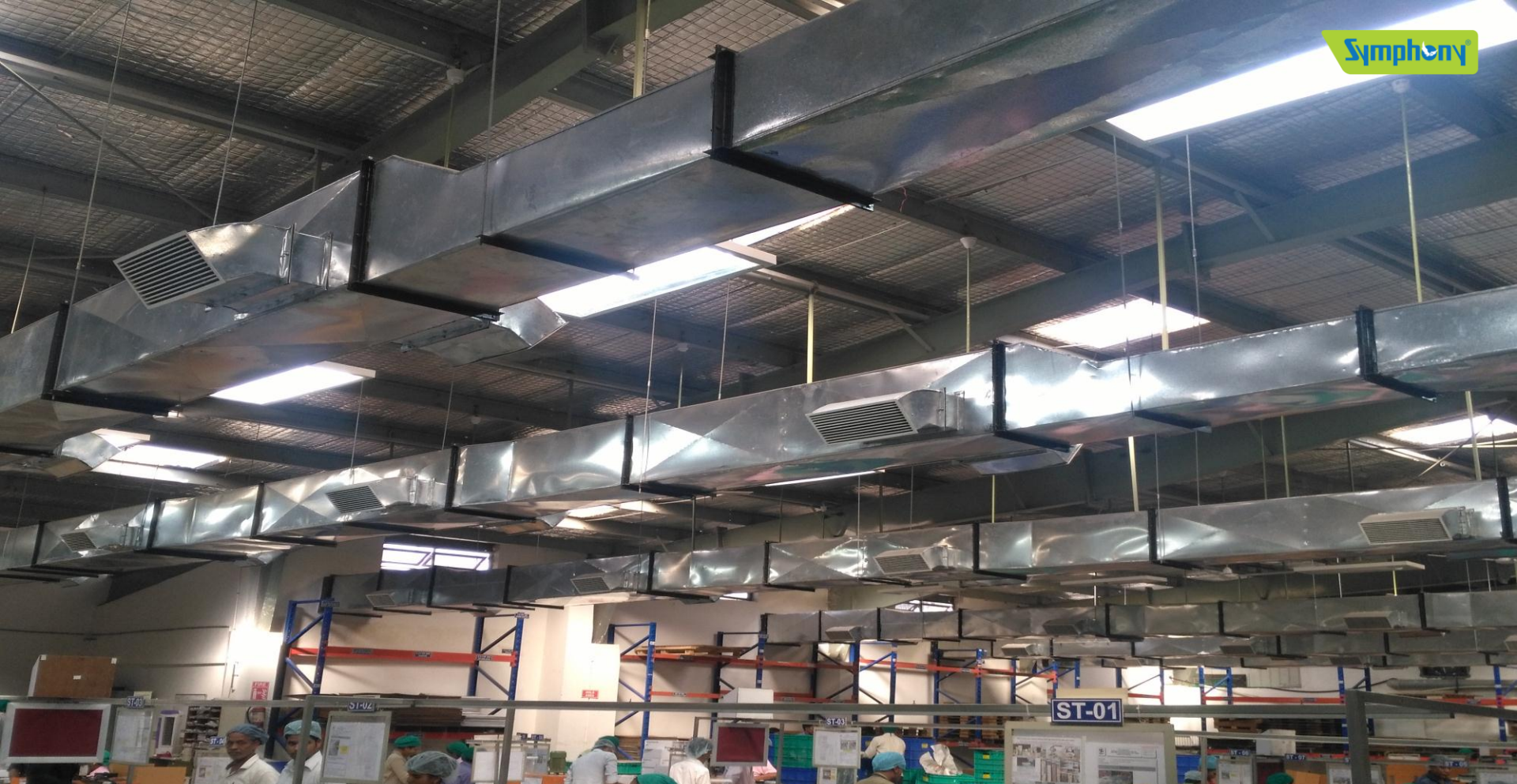
Ducting – All machines are connected to 80 feet duct having 10 outlets.
