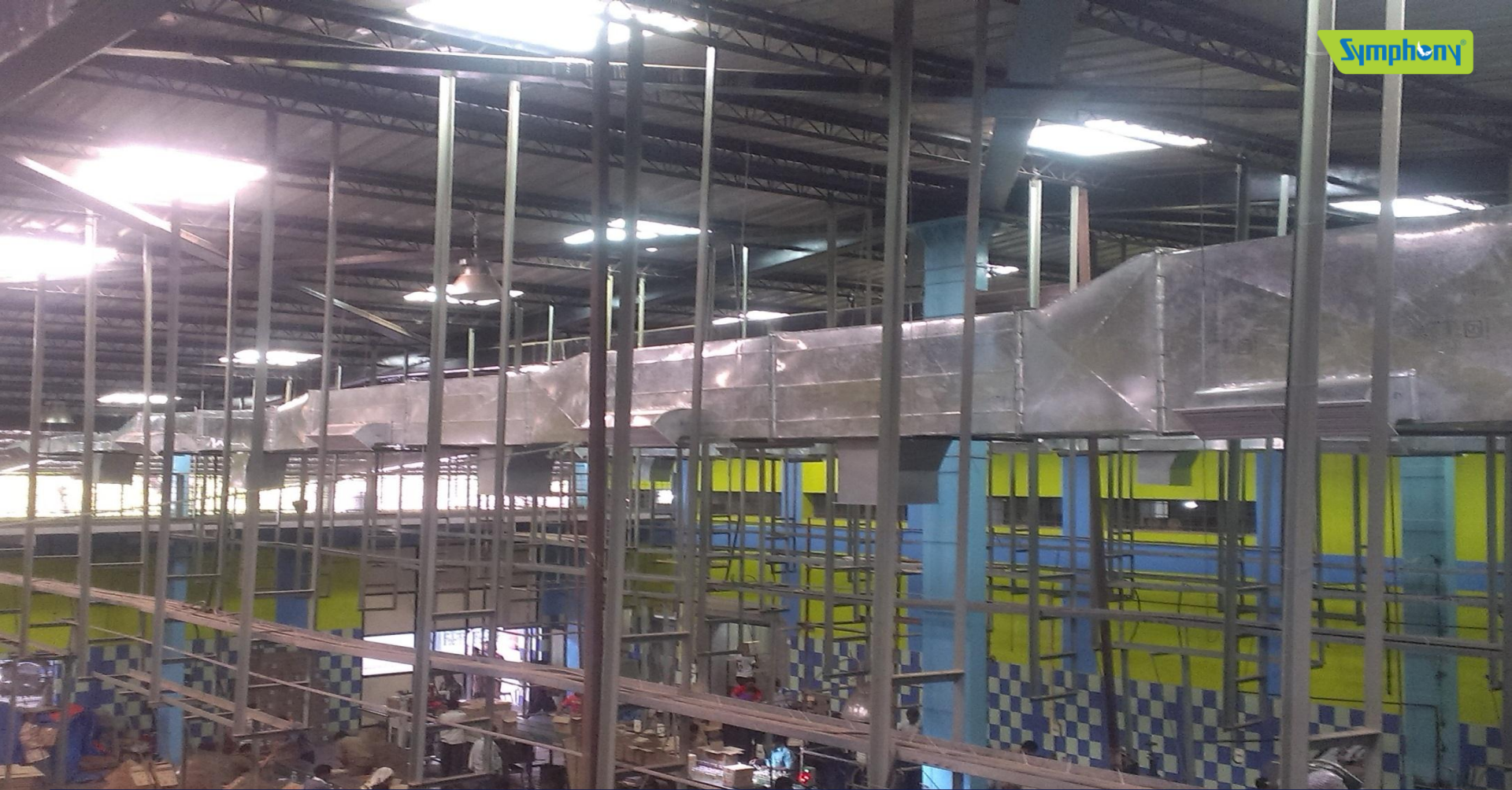
Ducting – Machine is connected to 200 feet duct having 36 outlets.
